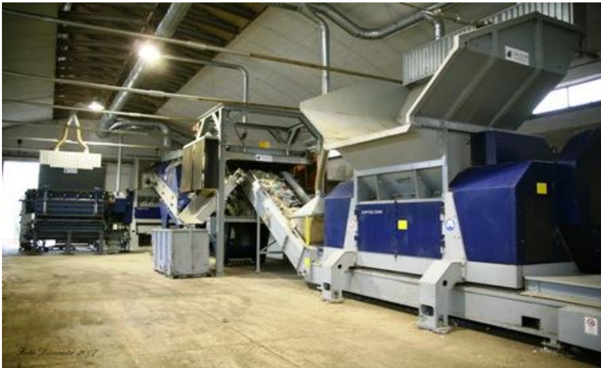
Picture 1: Plant for production of alternative fuel, Dalena Ecology Ltd
